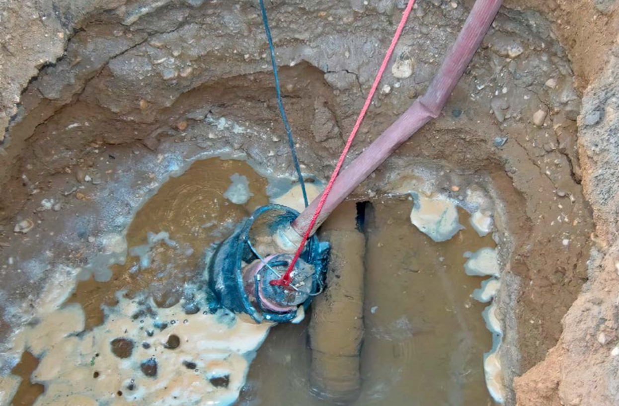
Figure 1. Example of a leakage in a cooling water pipeline.
